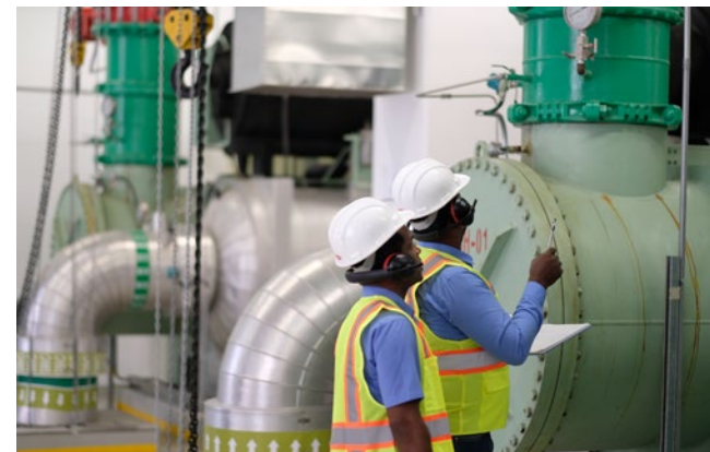
Cooling systems at Emicool
