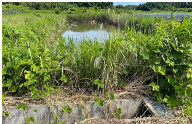
Drainage system (channels and ponds) at solar site of Nozomi
